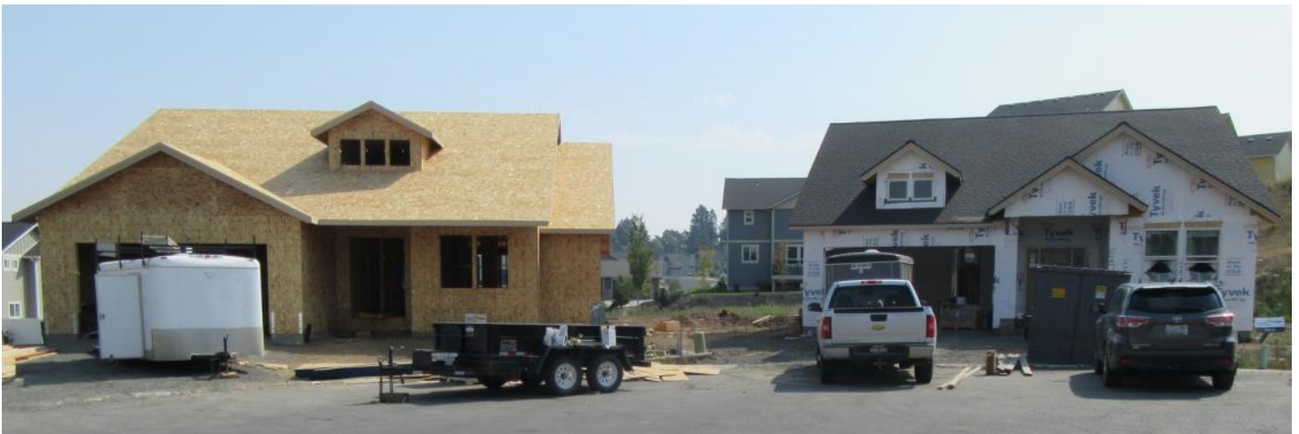
The pace of single family house construction on Sunnyside Hill seems likely to continue for the foreseeable future.
