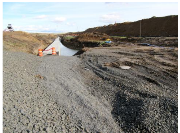
A view of construction west of the airport runway. The box culvert is shown on the left side of this photograph.
